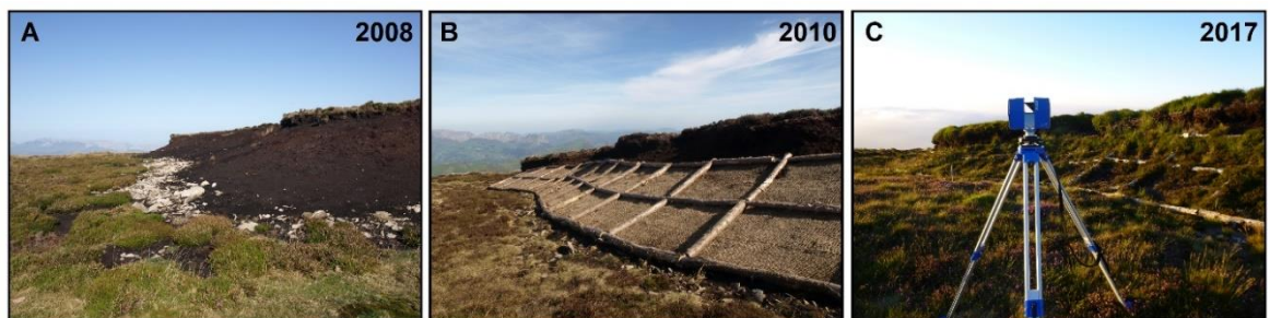
Figure 2.21. A) Exposed peat area at Zalama blanket bog (Photo: DFB); B) Geotextile example covering exposed peat surface at Zalama blanket bog (Photo: DFB); C) Area of exposed peat after restoration actions using geotextile.
