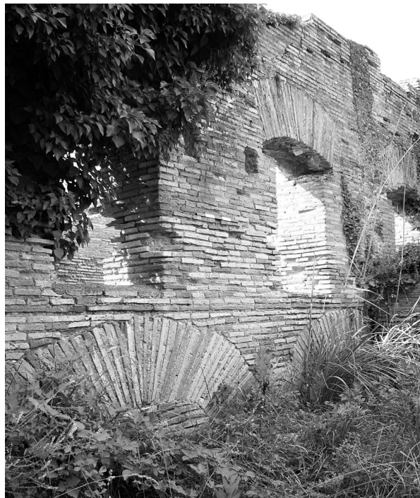
Fig. 5.57 – A row of arches reinforces the western wall and counteracts the sloping terrain
