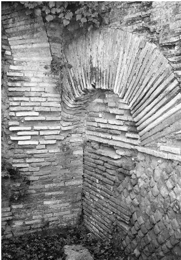
Fig. 5.59 – Reinforcing arch placed to strengthen the joint between the earlier opus reticulatum (brick) and the later opus latericium walls
