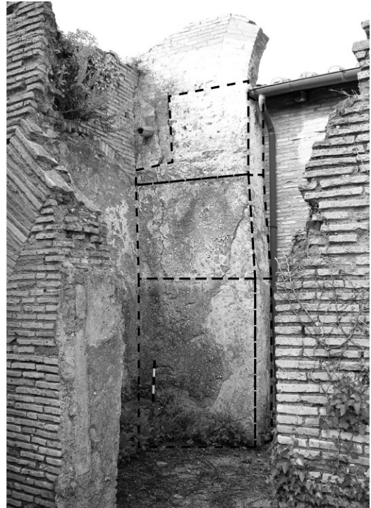
Fig. 5.15 - Travertine blocks forming the arched door opening of the preceding building, integrated into room 08 which served as a small frigidarium of the later baths
