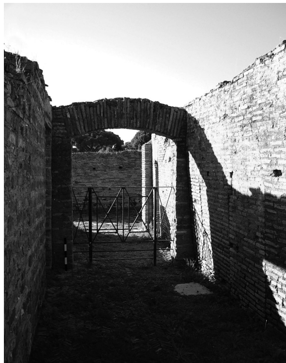
Fig. 5.62 – The main entrance to the Caupona, closed for visitors; the arch is a later intervention to provide structural support; the corridor is paved with opus spicatum (small tiles laid in herringbone pattern)
