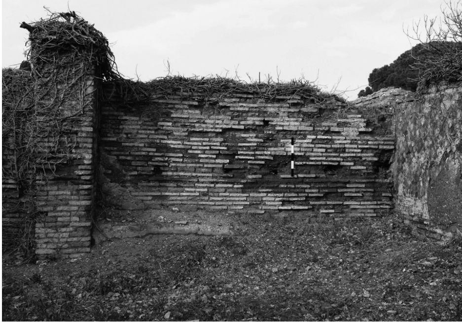
Fig. 5.31 - Partition wall placed against earlier opus reticulatum (brick) walls; the partition wall subdivides room 12 into tabernae on the cardo and changing rooms serving the baths
