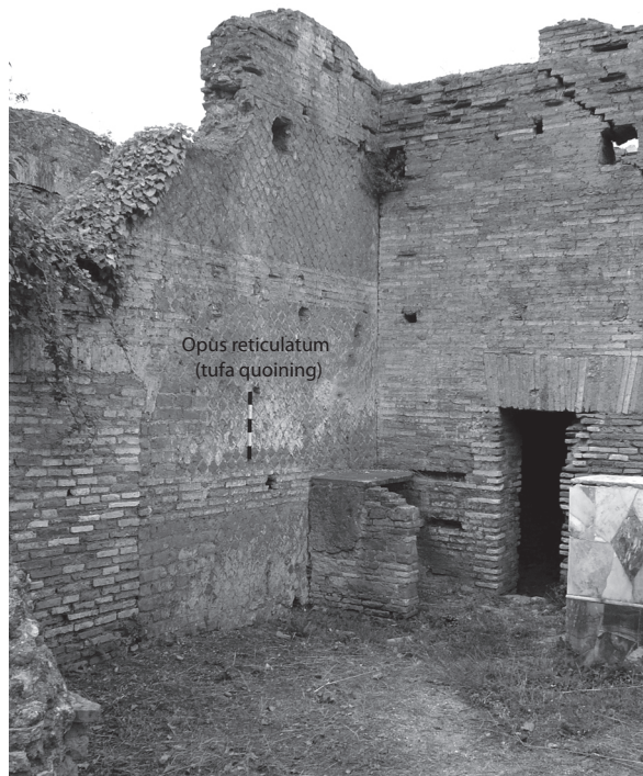
Fig. 5.30 – Earlier opus reticulatum wall integrated into the later structures; the walled-up door opening (left) had its lintel cut back to fit the higher floor levels (south-western corner of taberna 03, s. plan of the Caseggiato dell'Ercole Fig. 5.35)
