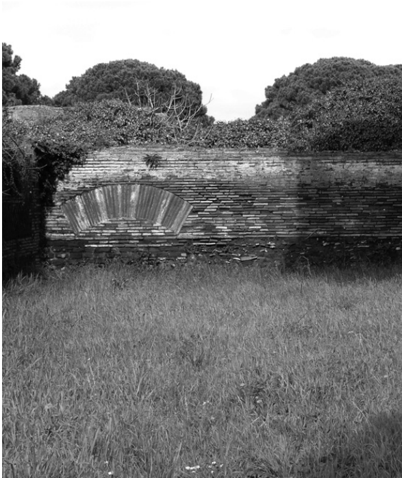
Fig. 5.81 – Caseggiato IV ii 9, retaining wall towards the southern 'open' space; the arch reinforces the construction against the Caseggiato IV ii 7
