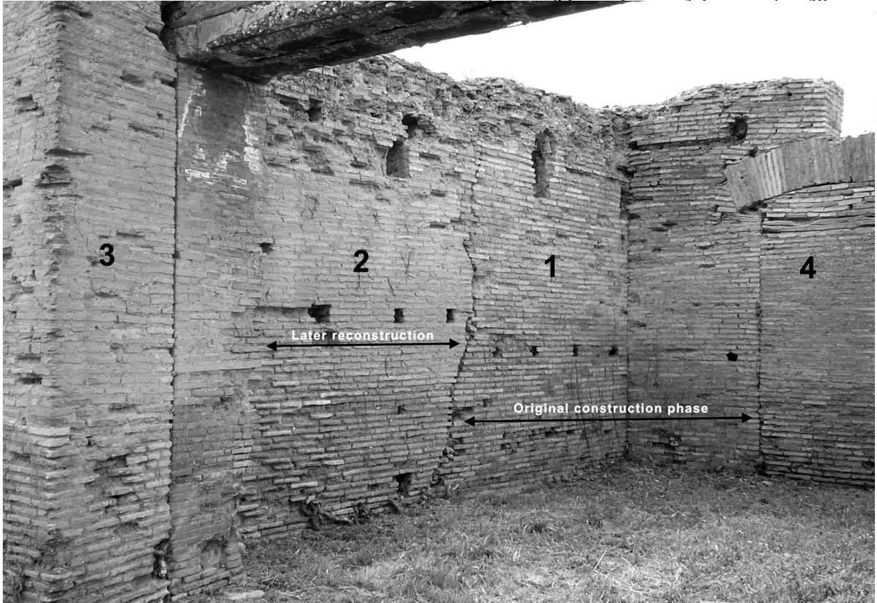
Fig. 5.43 – Room 10: 1) The original caseggiato walls (putlog holes at h 1.25 m; on top of bonding courses); 2) A later intervention, with putlog holes at h 1.50 m; 3) Reinforcement of the portico; 4) Walled-up door
