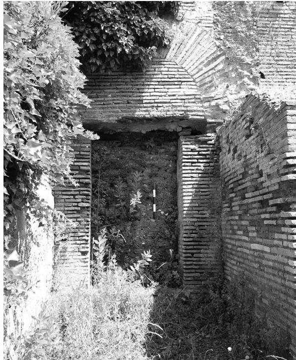
Fig. 5.56 – Former door leading to the open space in the north, closed by the water cistern serving the baths
