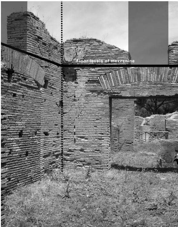
Fig. 5.42 – Door openings on the mezzanine upper floors are still preserved and are visible above the ground floor doors
