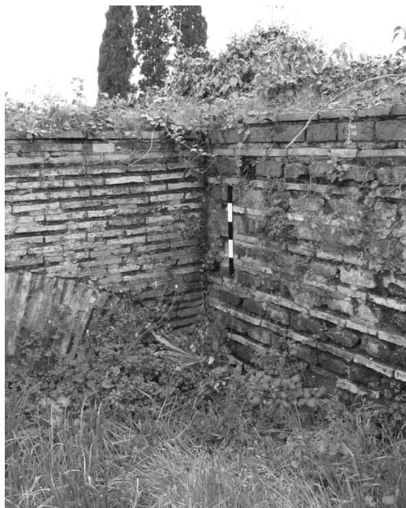
Fig. 5.75 – The south-eastern wall of the Caseggiato IV ii 7 precedes Building IV ii 9; photograph taken within Building IV ii 9 in its south-western corner
