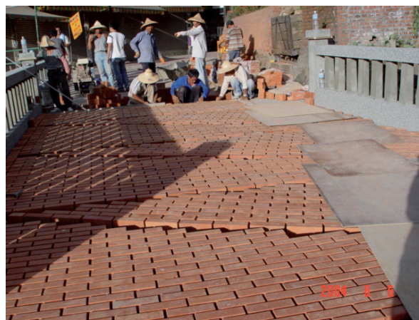
Fig. 3.3.9 Renovating the memorial Red Road (hong malu 紅馬路) next to the Siliandong. Photo was taken by the author in 2004.
