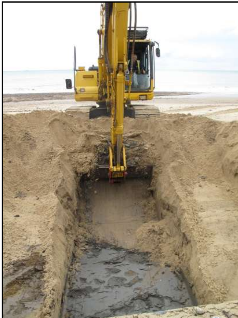
Figure 8 - Mechanical digger used to expose and excavate the deposits in the 2011 excavation by Leiden University (Photo courtesy of H. Kamermans).
