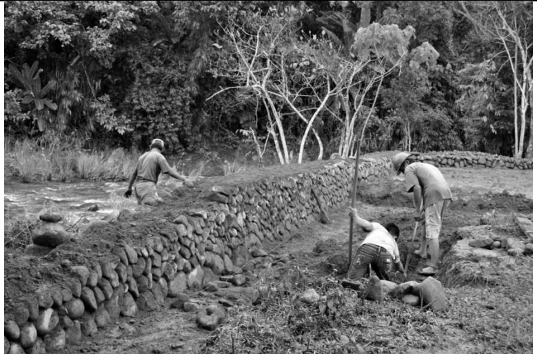
Figure 2: Ifugao people building a rice terrace in Diwagden, San Mariano (Photo by E.J. Versteeg 2015).
