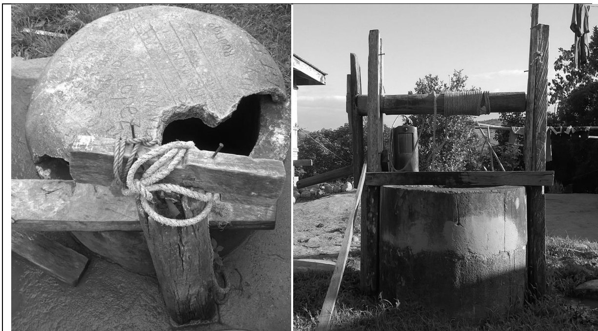
The damaged pump well of Purok 7. (Photo by J. Csala 2016)
