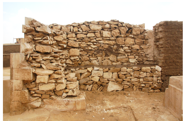
Fig. 34: North face of the pylon of Horemheb's tomb, with the strengthened rubble fill. Photo by Nicholas Warner/Leiden-Turin Expedition to Saqqara.
