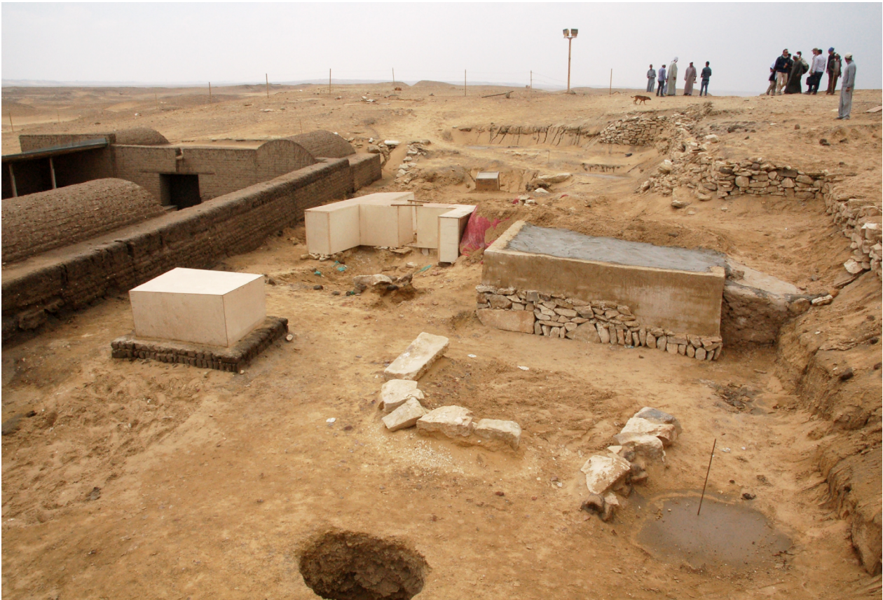
Fig. 35: The new protective covers devised for the Ramesside chapels found during the 2017 and 2018 seasons. Photo by Nicholas Warner/Leiden-Turin Expedition to Saqqara.
