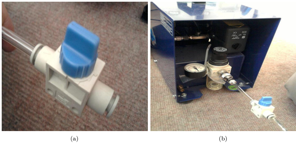
Figure 2.6: Air compressor connected with a switch where (a) is a connecting valve and (b) shows overall connection with air compressor.
