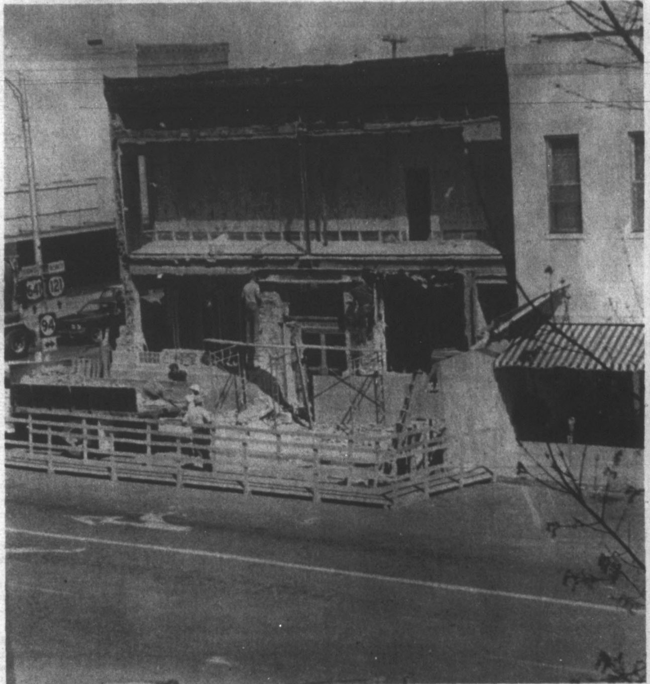
FACELIFTING — Facelifting is well underway at the Bank of Murray where workmen have torn off the front of the building facing Fourth Street. When completed, the older portion of the bank will sport the same facade as the new addition which has just been completed. The bank is providing all of its regular services in the new addition while the refurbishing of the older portion is being completed. Bank officials predict the project will be finished in six to eight months.
