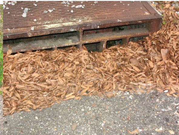
Storm Drain (rating 2) semi-blocked
