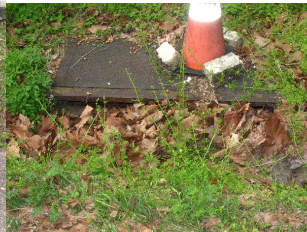
Storm Drain (rating 3) blocked
