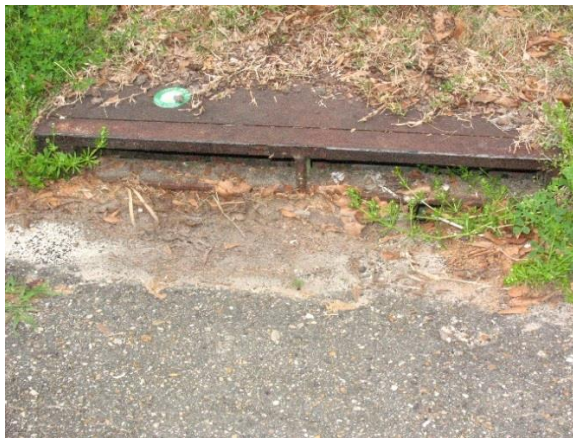
Storm Drain (rating 2) semi-blocked
