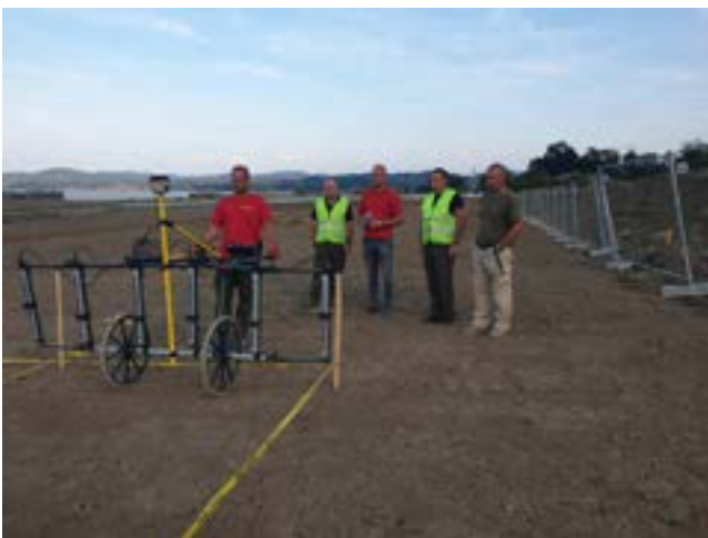
Photo 2: Use of devices that allow the application of a passive and active method on ERW clearance project related to Data Center construction site in Kragujevac
