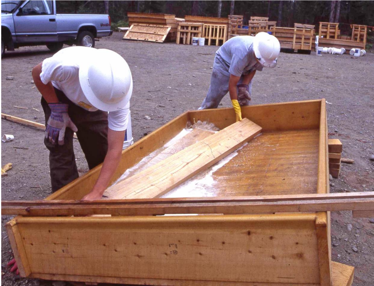
Fig. 16. Dipping section joists in wood-preservative in fiberglass-lined wooden “bathtub.” Components of interpretive stations (Fig. 8) appear in background along with full and empty 5-gallon buckets of wood preservative. Tom Hanson’s truck is in left background. Ronald B. Davis photo.
