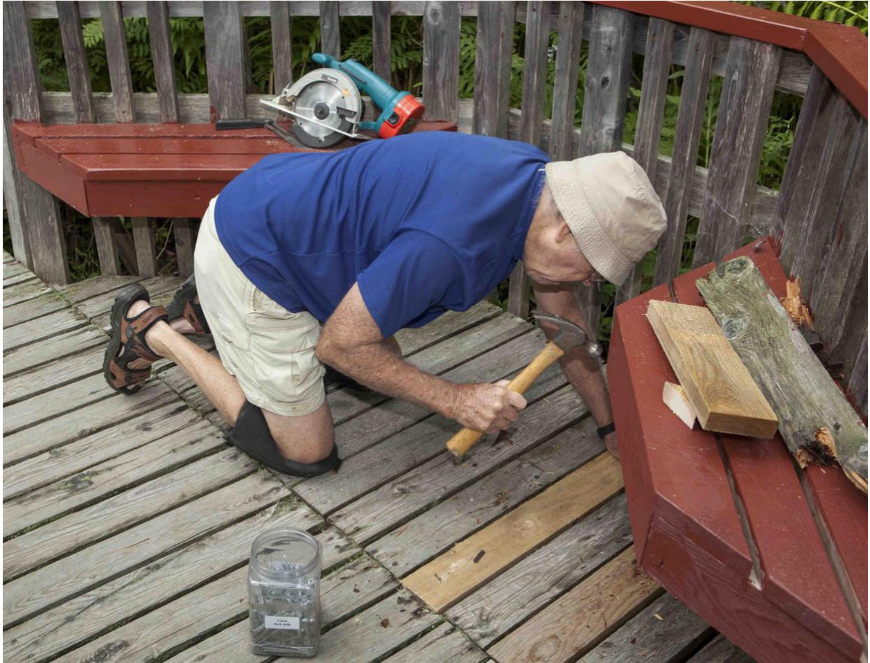
Fig. 29. Phil Locke replacing a broken deck board at IS1 on 13 August 2012. Ronald B. Davis photo.
