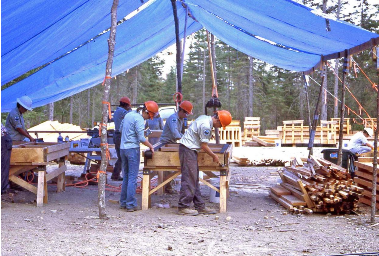
Fig. 15. Maine Conservation Corp crew members at assembly site in summer 2002. Member in central foreground is spiking an end joist on a boardwalk section (see Fig. 6) using a small sledgehammer (zoom in). The incomplete section rests in a jig supported on sawhorses. 45 An incomplete section in another jig is at far left. Its middle joist is in place. The heads of three spikes can be seen on the end joist (zoom in). A pile of bump railings is on the right. Stockpiled components of interpretive stations including railings (see Fig. 8) occupy right background, and a pile large dimension lumber rests in far left background. Ronald B. Davis photo.
