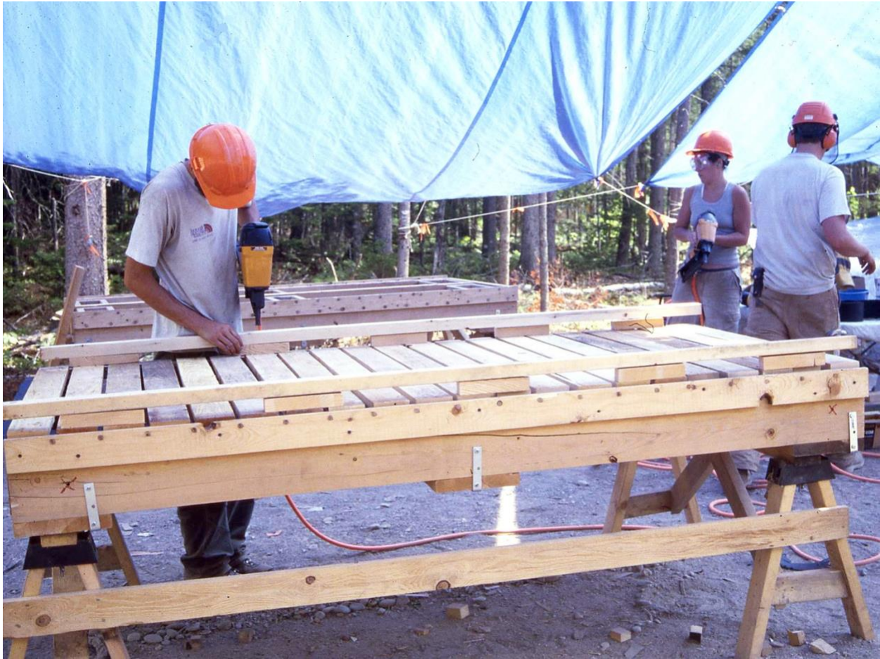
Fig. 17. Final stage of assembling a boardwalk section in the jig in the foreground. 45 An MCC member is nail-gunning a bump railing atop riser blocks at the ends of the deck boards. On the closest face of jig, the insertions of the half-inch diameter pegs used to space apart the deck boards can be seen. The jig in the background contains a section's longitudinal joists with end joist attached on the right, with the left end joist leaning against the jig. Ronald B. Davis photo.
