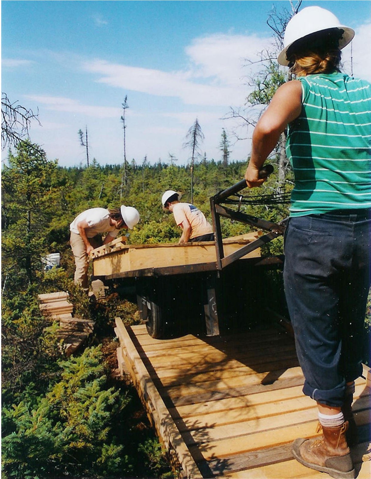
Fig. 20. MCC member tipping/sliding section off cart at end of incomplete boardwalk onto composite footings. Ron Lisnet UM photo.
