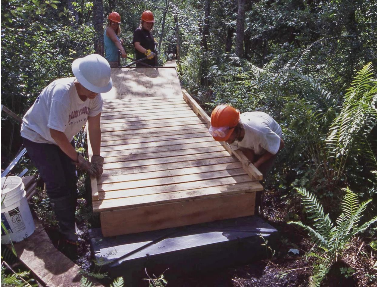
Fig. 21. Receiving section from cart at end of incomplete boardwalk and positioning it onto floats in mid-summer 2002. This location has standing water in spring. Ronald B Davis photo.
