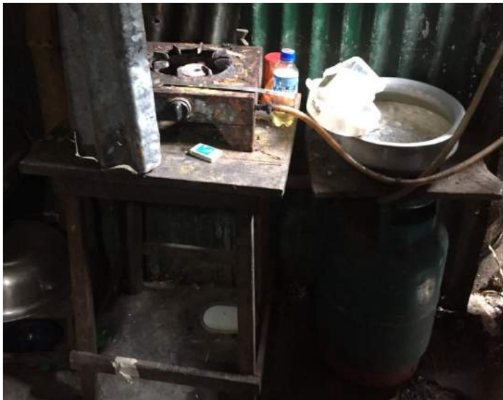
Figure 7.15: Gas cooking arrangement (M Jones)
