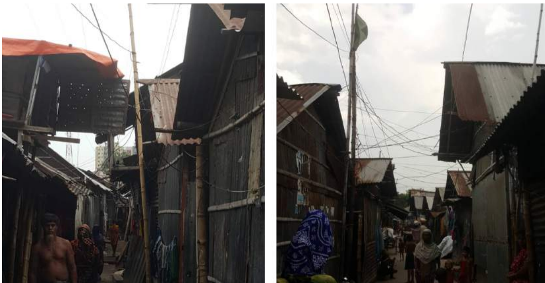
Figure 7.6: Bamboo electrical poles (S. M. Younus)
