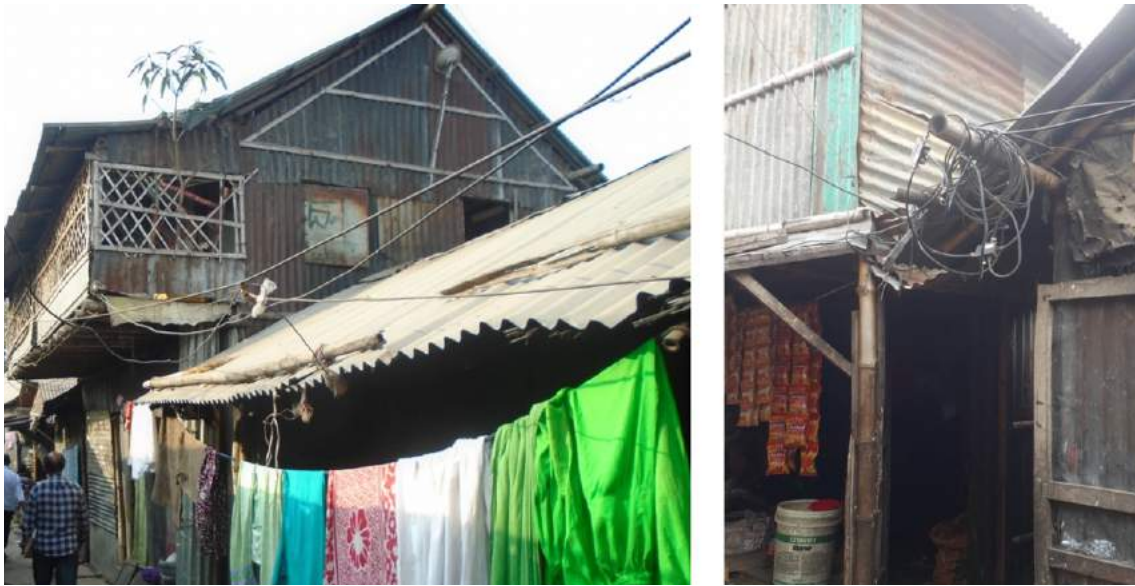
Figure 7.5: Unsafe electrical cabling (M Jones and S. M. Younus)
