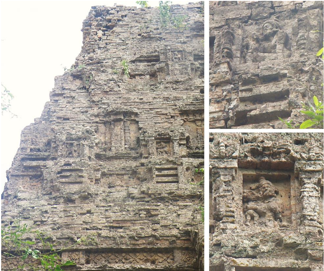
Figure 5.45 Superstructure of S1, Sambor Prei Kuk, with representations of populated architecture. Photographs: Author.
