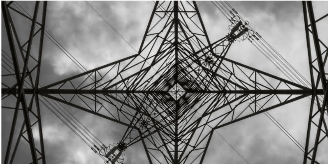
Electricity pylon in Sussex, UK, Credit: sagesolar (CC BY 2.0)
