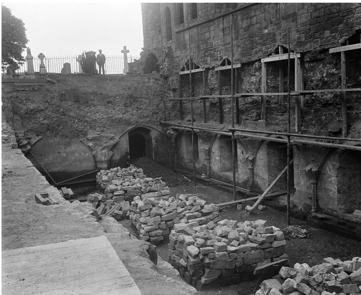
Fig 100: Excavation of the refectory of Dunfermline abbey in 1900 - c.1560 - was such a domestic, non-sacred structure a possible source of stones for an improvised crypt for the 'Bruce grave'?
