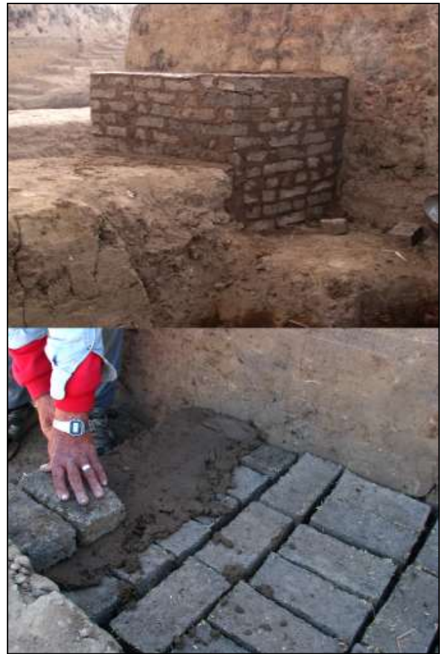
Figure 6: Construction of mudbrick wall as an addition to mastaba (photographs by authors).
