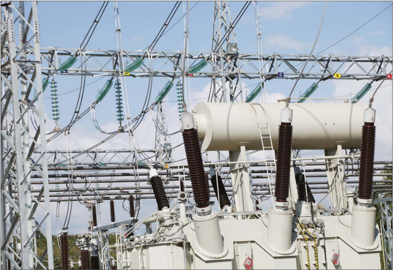
Figure 4. Power transformer bushing
