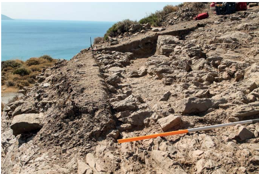
Figure 11. Final Neolithic retaining wall (un. 267) visible on both sides of N baulk of Trench 12; north face damaged by bulldozing of A1 road (from NW).
