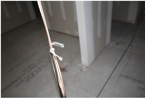
(e) Kitchen Gas Intake
