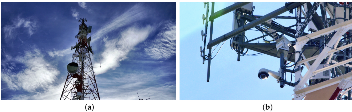
Figure 7. Surveillance system located in a telecommunication tower (Telefónica Digital España).
