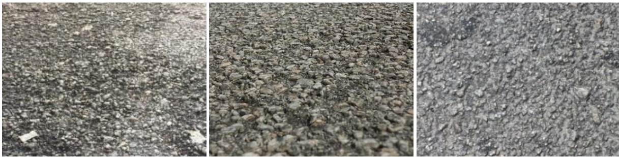
Photo. 1 – Wash-out detected on the asphalt pavement surface
