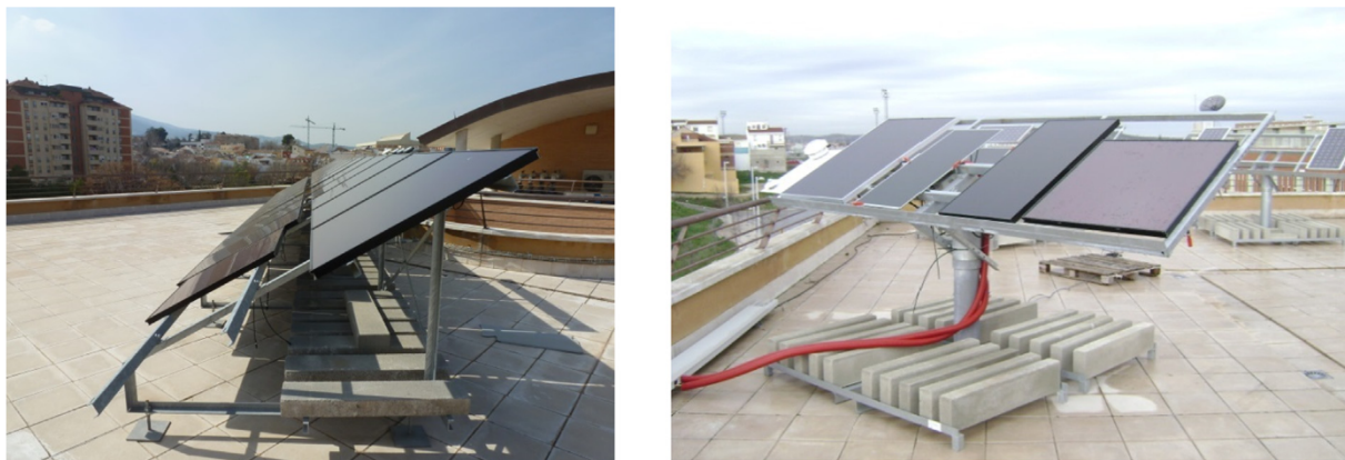
Fig. 1. Photographs of the PV specimens investigated over the course of the experimental campaign. Left: PV fields of PVGCS #1 (a-Si, upper row) and PVGCS #2 (a-Si/ \mu c-Si, lower row). Note that the a-Si PV module closest to the viewer in the lower row does not form part of PVGCS #2. Indeed, such PV module was left in open circuit conditions for other research purposes. Right: PV modules tested and measured (from left to right: a-Si/ \mu c-Si, CdTe, CIGS and a-Si).
