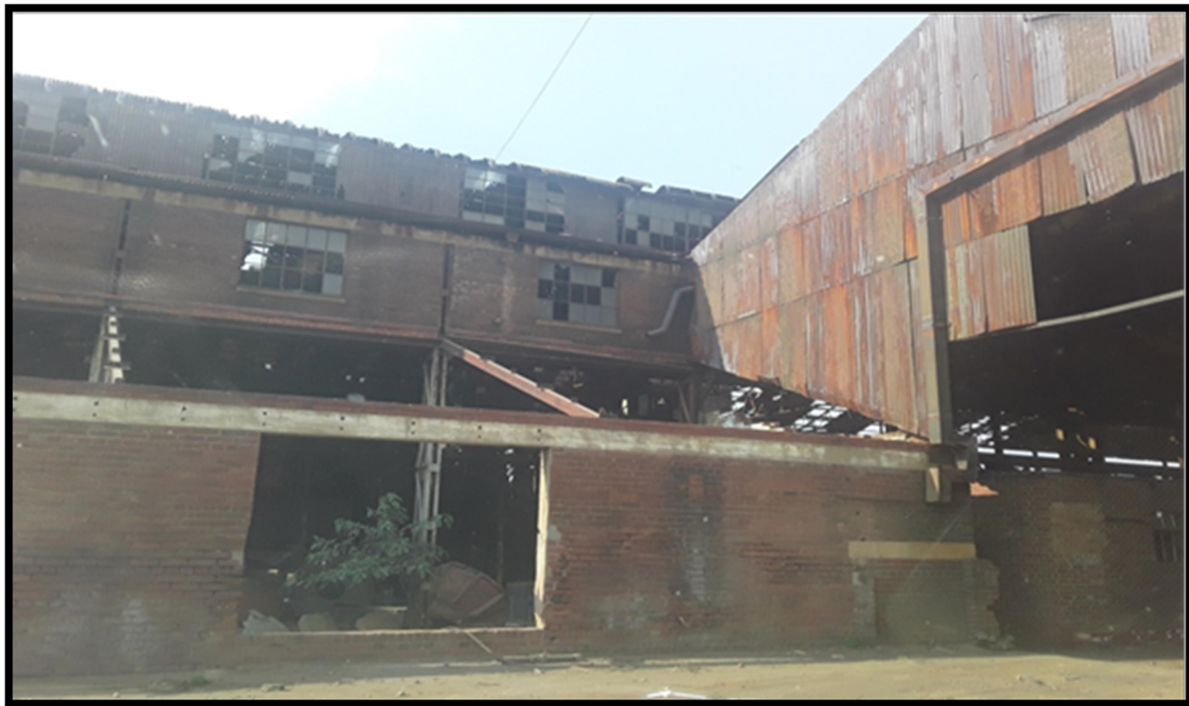
Figure 6.4 Dilapidating industrial building in Bulawayo
