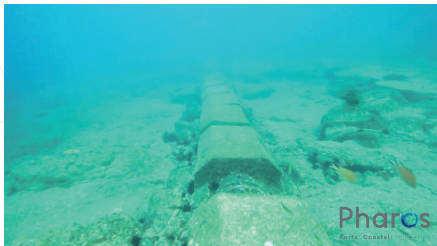
Figure 22. Detail of the concrete weights in a pipeline section near the coast.
