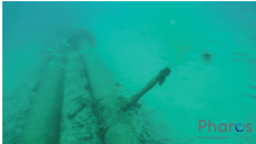
Figure 20. Detail of the diffuser system of the submarine emissary pipeline.
