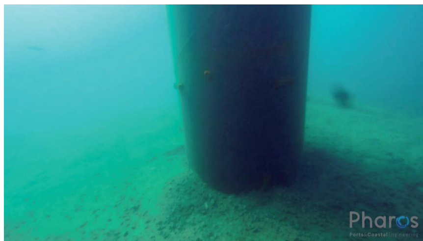
Figure 26. Detail of upper surface and pile in the foundation of the Duke of Alba (Port of Naos).
