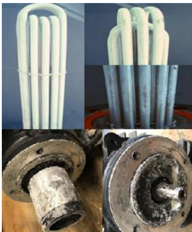
Figure 4-13 Formation of scale on reboiler bundle and pump head
