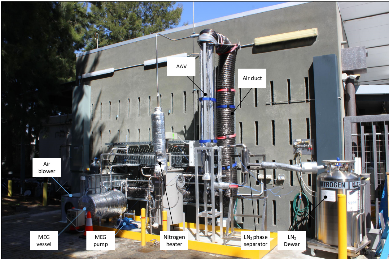
Figure 7-6. Site photo of the system of ambient air vaporizer
