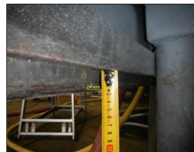
(f) Legged tank settlement: Less than 1% in 2013
