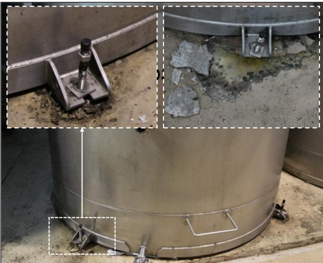
(c) One loose bolt resulted in damage to the concrete slab and the other loose bolt caused no visible damage to the concrete slab
