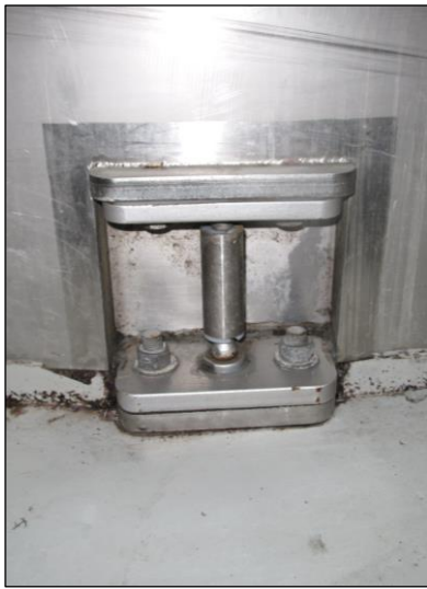
(a) Energy dissipation devices used for anchoring 40 kL tank
