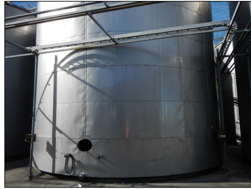
(d) 550 kL tank - minor damage to the barrel
