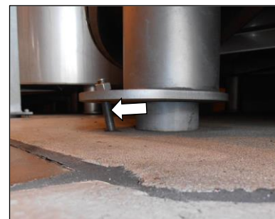
(c) Anchor bolt damage: 1.0% in 2016
