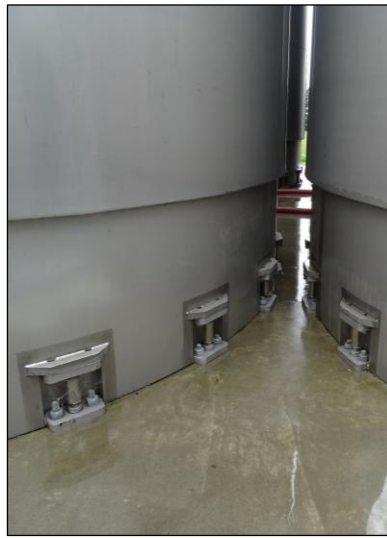
(b) Energy dissipation devices used for anchoring 120 kL tank
