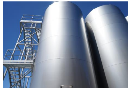
(c) 90 kL tanks, after 2016 earthquake
