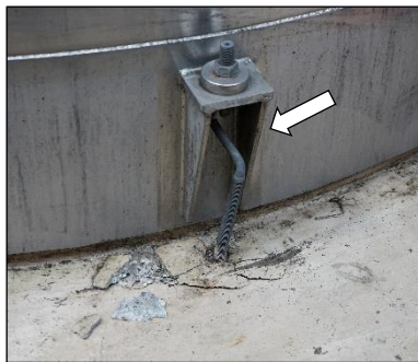
(a) Bolt buckling: 6.1% in 2016
