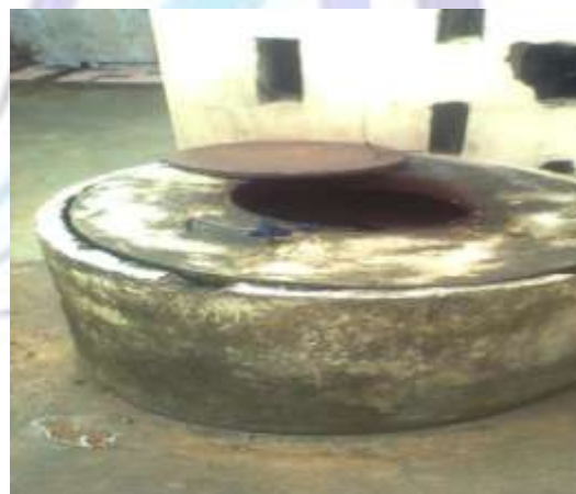
Well F: A raised well with metal cover constructed closed to a generator house
