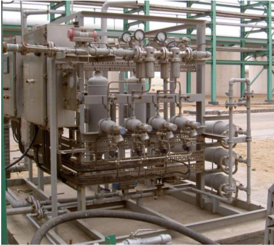
Figure 7: Nitrogen Generation Package
