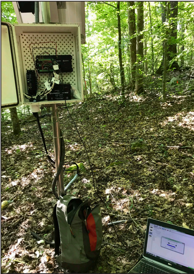
Figure 6. Example of a field station at the Roberts Bend landslide. The enclosure contains a data logger and battery, which is charged by a 10-watt solar panel.
