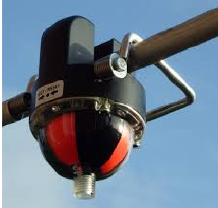
Figure 3.2: Fault Passage Indicator.
