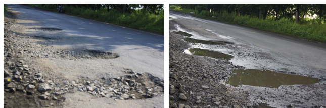
Fig. 1: Potholes on Indian road: dry (left) and water-filled (right)
