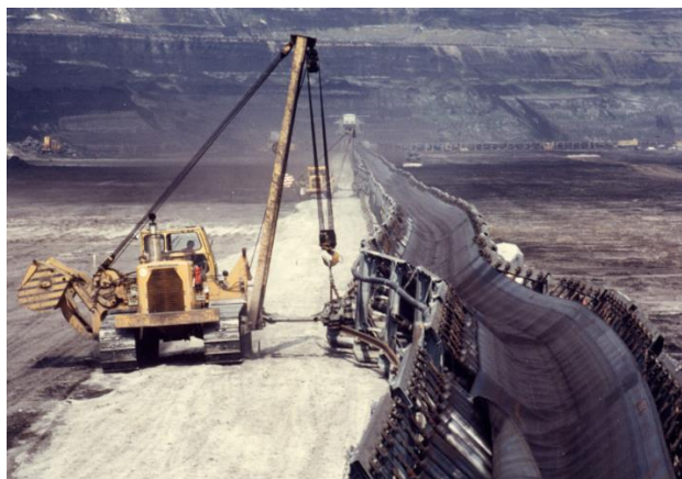
Figure 2-8. Shiftable conveyor belt installed at the operating face [52]
