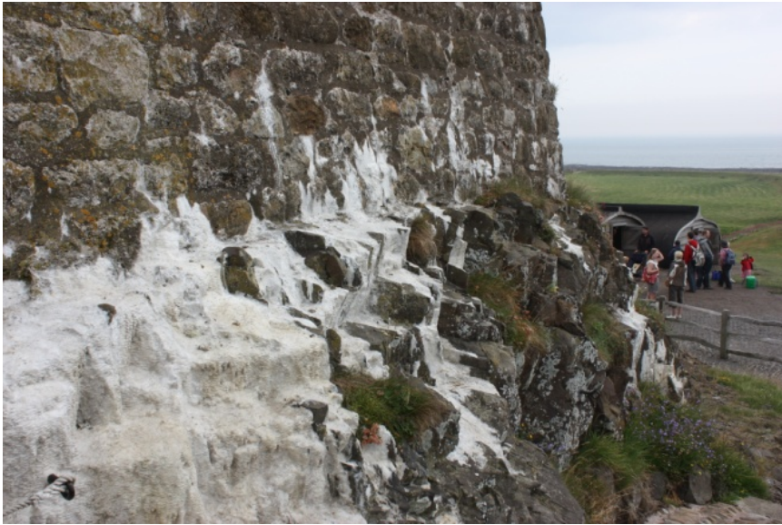
3 4 Fig. 1. Speleothem (flowstone) attributed to carbonate leaching from lime rich mortar, 5 Lindisfarne Castle, Northumberland, UK.
