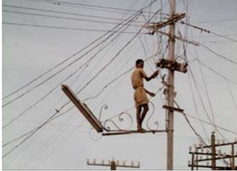
Figure 1.2: A photograph showing a person hooking wires to the distribution lines to steal power
