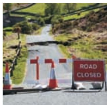
GeoHazarD: dormant landslide reactivated after a rainstorm, resulting in a road being cut near Ainthorpe on the North York Moors.
