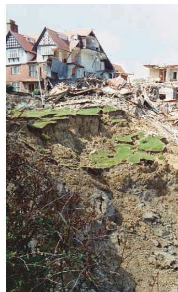
GeoHazarD: a large slump in glacial till led to the destruction of the Holbeck Hall Hotel, Scarborough, in June 1993.
