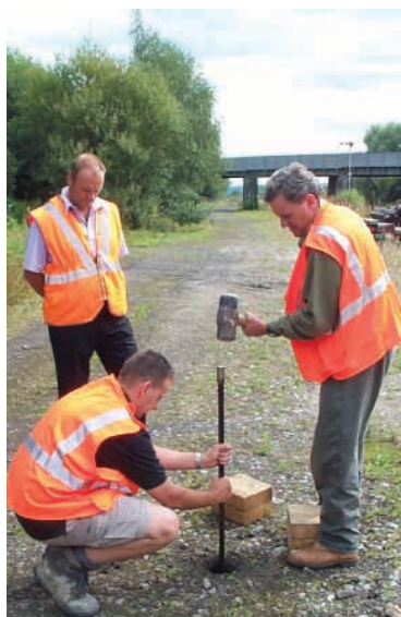
Assessment of railway trackbed performance: testing the ballast and subgrade at Leominster railway station.
