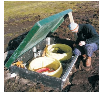
National earthquake monitoring: a new broadband seismometer station installed at Lerwick Observatory, Shetland.
