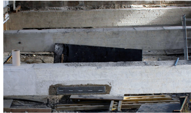
Figure 13: Textile sensor applied in the concrete beam of hydroelectric power plant.
