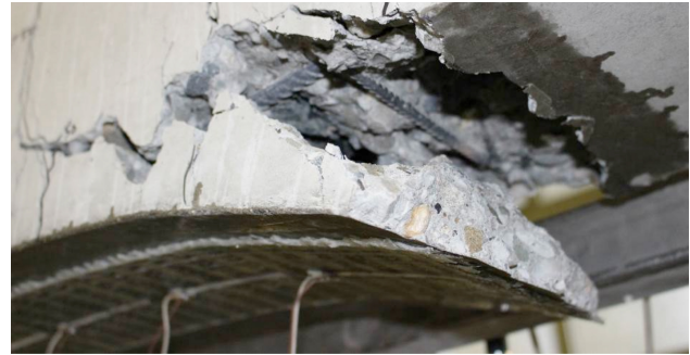
Figure 8: Failure of RC beam strengthened with Carbon Fibre Reinforced Polymer smart-textile.
