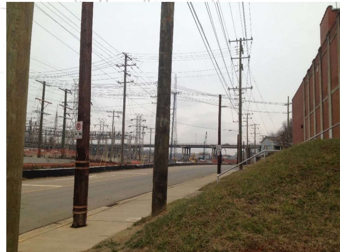
Duke Sub-power Facility
