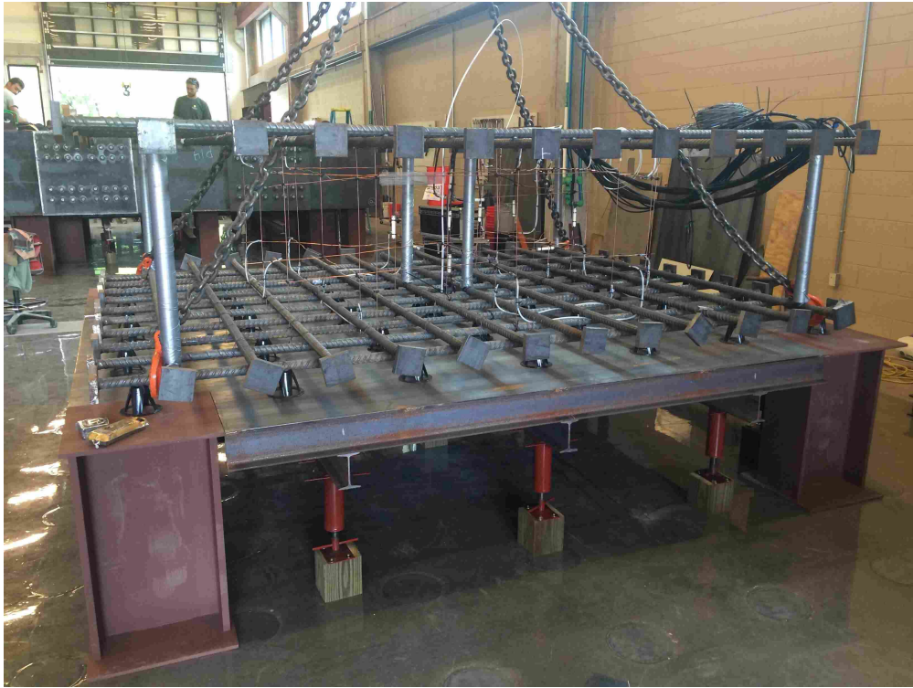
Figure A.5: Completed construction of the bottom formwork with cage in place
