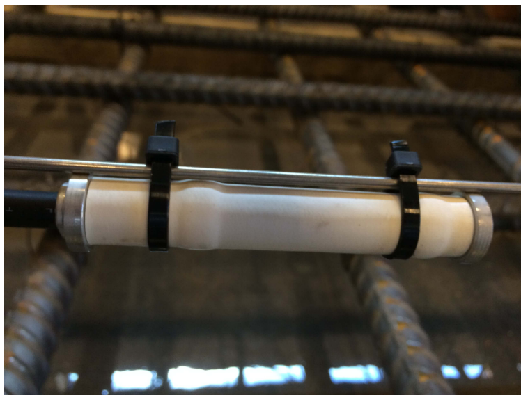
Figure A.9: KM-100B strain transducer attached to positioning bar within rebar cage
