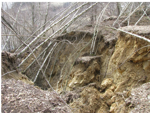
FIGURE 5. Significant radial cracks between two blocks of the central part of the rockslide
