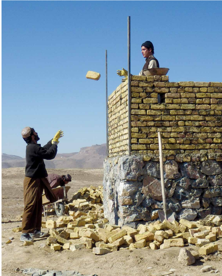
Afghan contractors help Afghan National Army soldiers build a latrine 7 February 2013 near Takir, Afghanistan. (Photo by 1st Lt. Gerrelaine Alcordo, U.S. Army)
