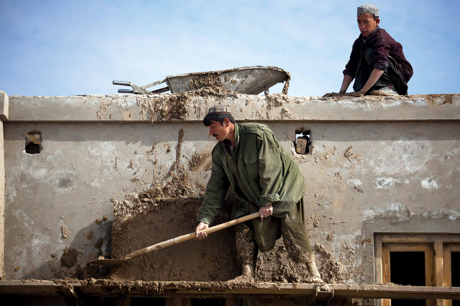
Afghan contractors reinforce the roof of a school under construction 19 January 2012 in Garmsir District, Helmand Province, Afghanistan. Twelve permanent schools were under construction by Afghan contractors in the Garmsir District. A civil affairs team in support of the 3rd Battalion, 3rd Marine Regiment, visited several of the sites to inspect the structures and ensure compliance with the quality assurance standards of the Afghan government. (Photo by Cpl. Reece Lodder, U.S. Marine Corps)
