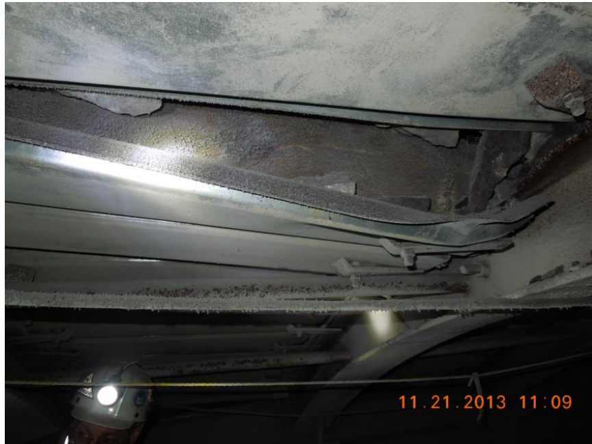
Figure 5.23 - Improperly installed lagging
