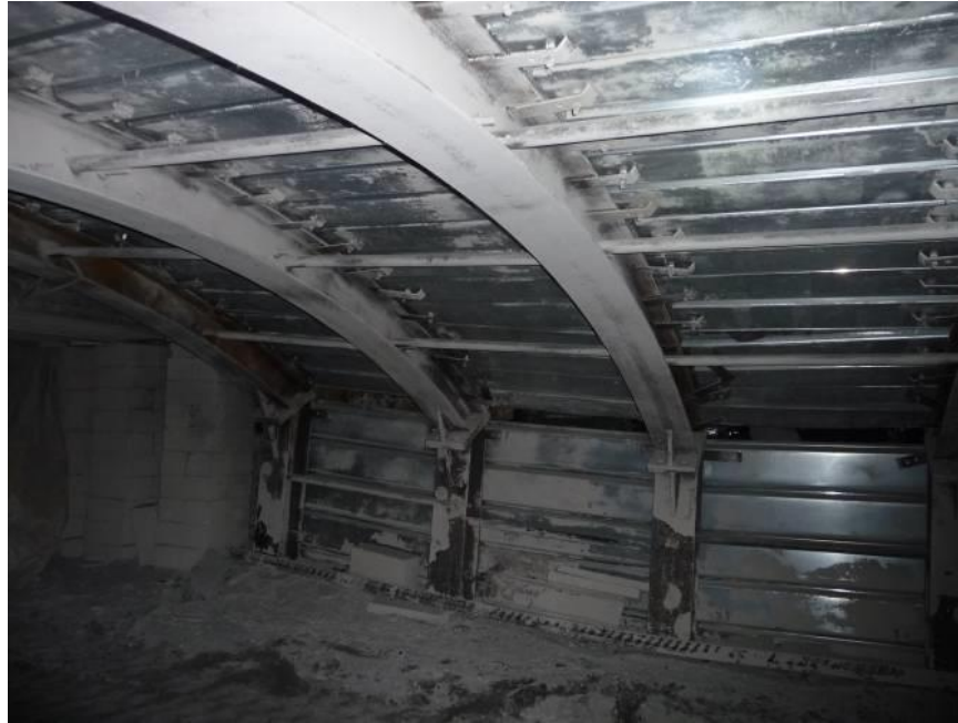
Figure 5.14 - Arch set and lagging impacted by roof fall
