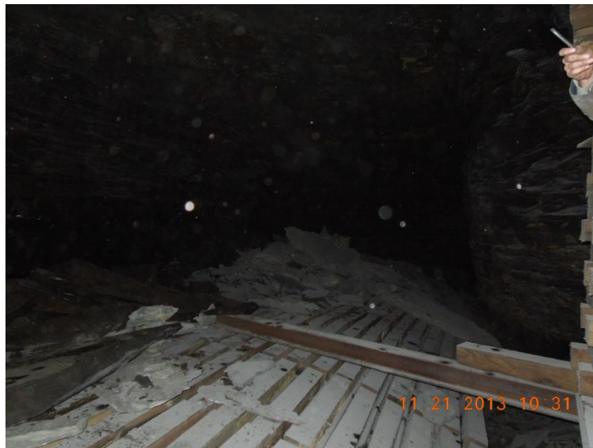
Figure 5.15 - Secondary roof fall
