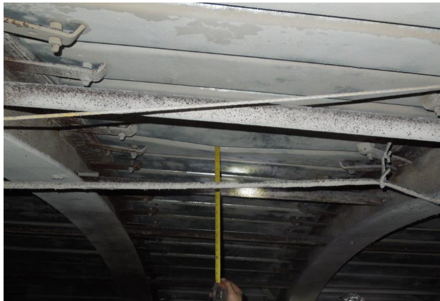
Figure 5.20 - Minor lagging deflection (0.25") due to rock impact
