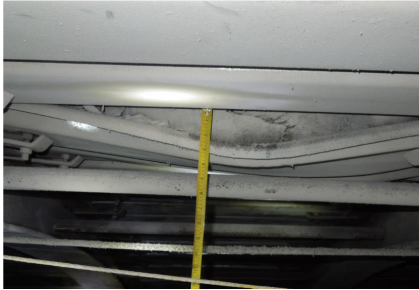
Figure 5.21 - Medium lagging deflection (3.5") due to rock impact
