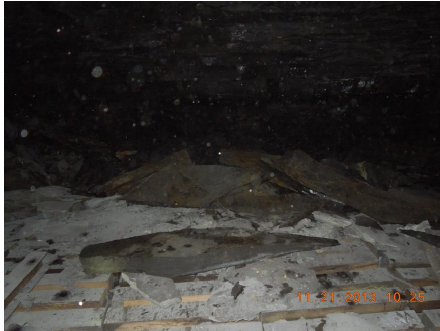
Figure 5.16 - Secondary roof fall
