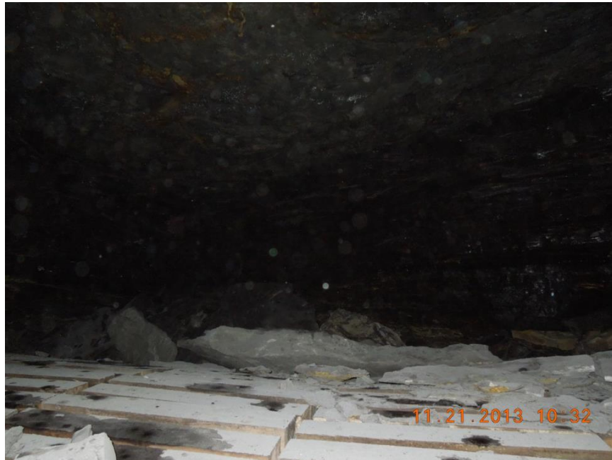
Figure 5.17 - Secondary roof fall
