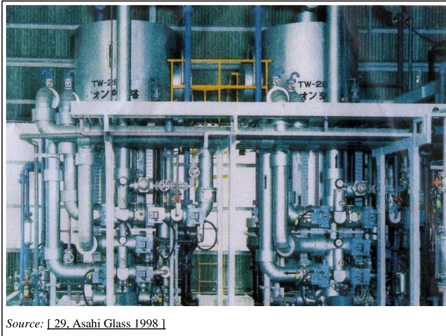
Figure 2.17: View of chelate resin towers in a secondary brine purification system
