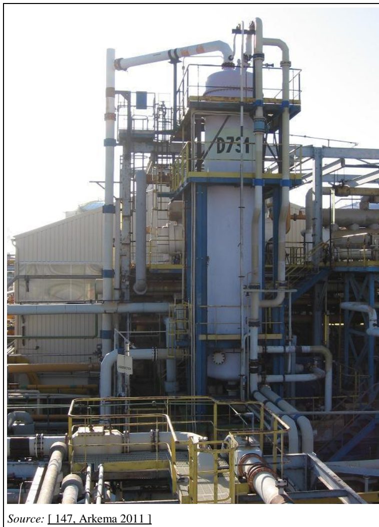
Figure 2.18: View of a chlorine absorption unit
