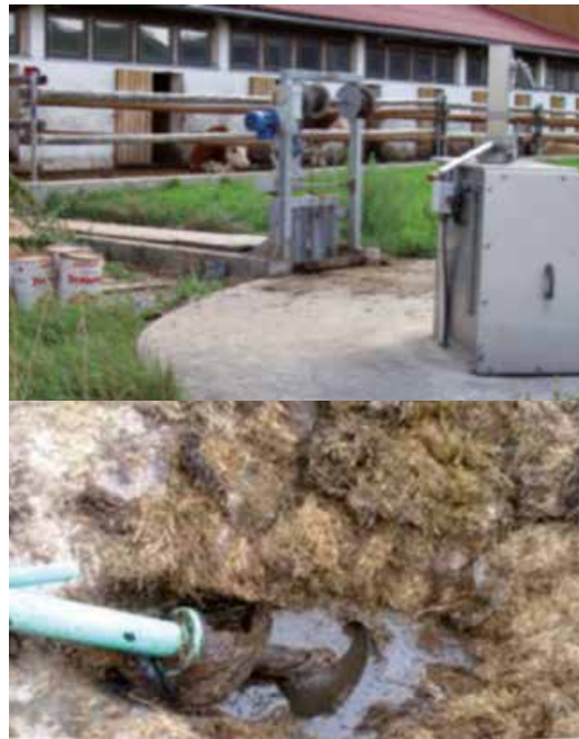
Figure 7 Digester feeding options; Gravity feed of manure into the tank – top photo: S. Baumann; Feedstock augered directly into a digester – bottom photo: A Bywater
