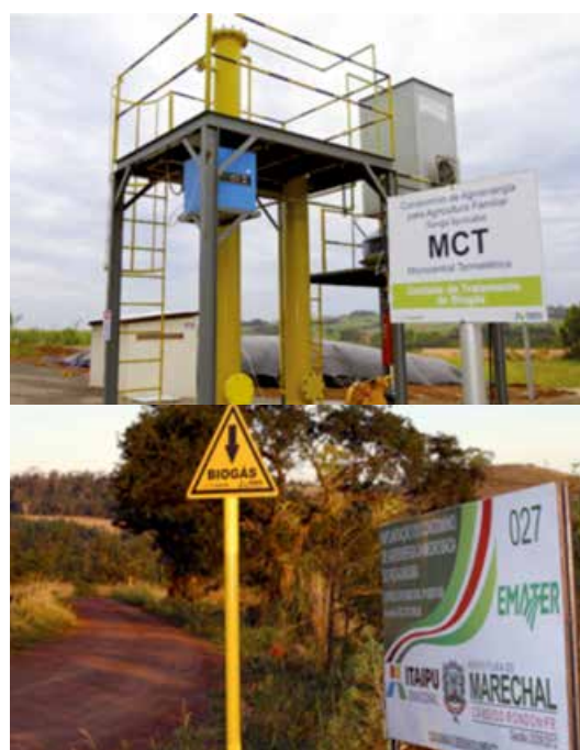
Figure 10 Small biomethane upgrading plant in Brazil; top: pilot biomethane upgrading plant which serves a co-operative of 33 family farms with an aggregate of 100 LSU, Capital cost: £66,000, Biogas throughput: 5 Nm 3 /hour (Photo: ITAPU Binacional, Brazil, 2014); bottom: biogas is transported through a pipeline to link the farms to a central CHP adjacent to the new upgrading plant.(Photo: Clare Lukehurst)
