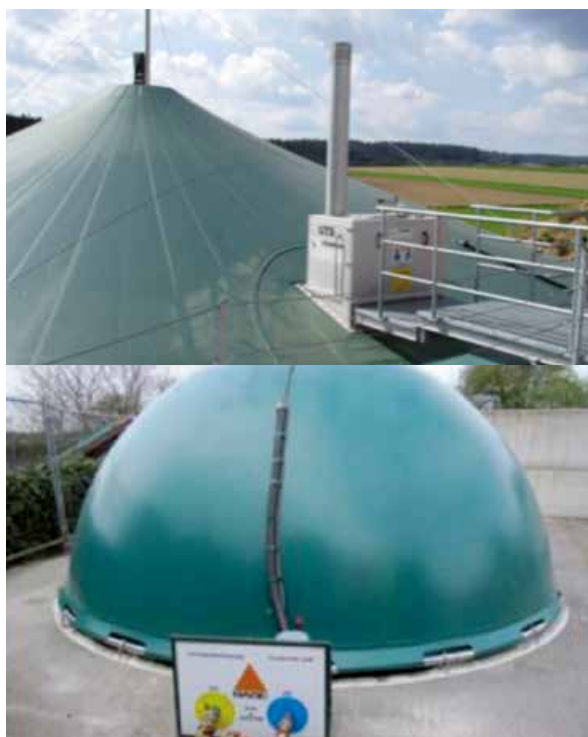
Figure 8 Gas storage in a flexible roof (top) and in a double membrane gas holder (bottom) (Photos: B.Drosg (top); A. Bywater (bottom))
