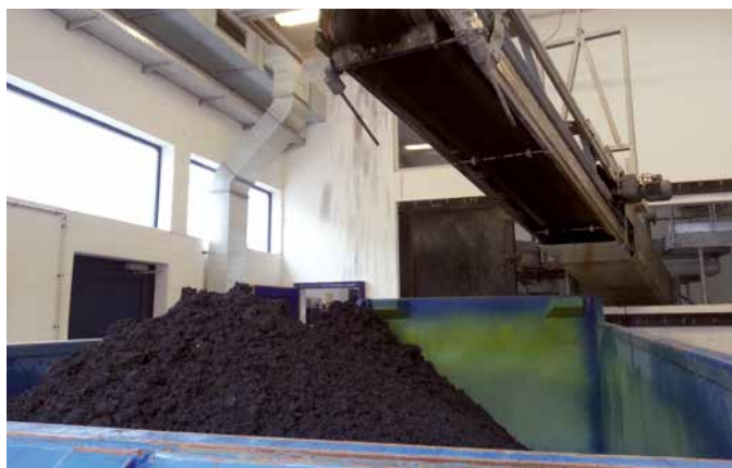
Figure 5: Dewatered sewage sludge
