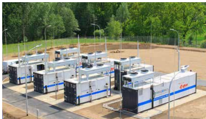
Figure 9: 2MW Power to gas unit based on alkaline electrolysis in Falkenhagen, Germany. The hydrogen is injected into the gas grid without methanation. (Source: E.ON)
