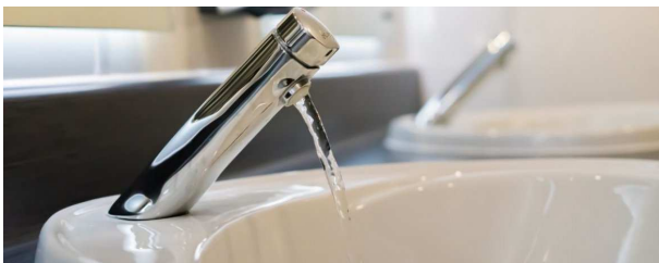
Figure 9. Push water taps (Commercial Washroom, 2019).
