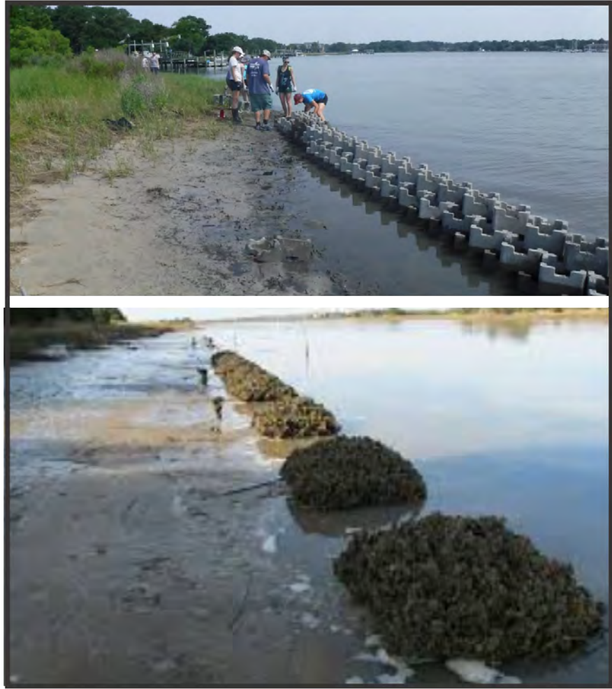
Figure 8. Example of oyster castle placement in an estuarine environment (Photo from Allied Concrete). The top image shows what the reefs look like when first placed. The bottom shows the reefs after oyster recruitment. The proposed structures for Hog Island are higher and wider than this oyster castle sill.
